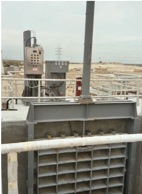
Waste Water Pumping Station, Alexandria, Egypt – 108" (2.7 M) x 108" (2.7 M) Cast Iron Sluice Gate with hydraulic actuation
