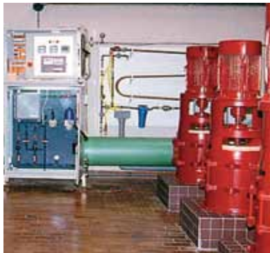
Automatic pump operating time recording using the Minilog B.
