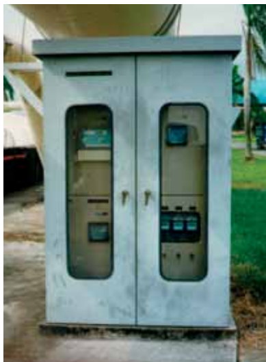
Four Minilog B devices record wastewater inflow on a large treatment plant in South East Asia.
